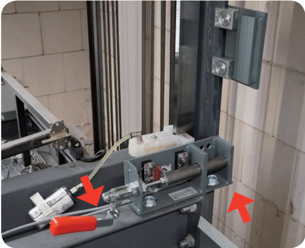
Release lever for the inspection travel is up, bolt is retracted
